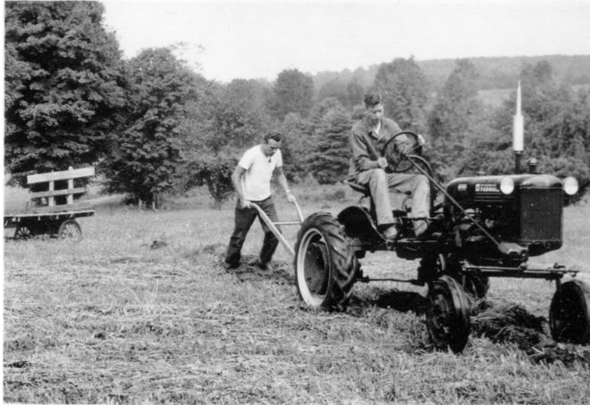
Bob Curran and Ken using hand plow to cut path for sewage distribution pipe
